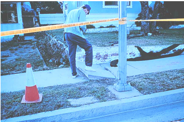
Fig. 3. Slab displacement due to permanent ground displacement. San Fernando valley, Calif. 1994 (Balboa Blvd).
