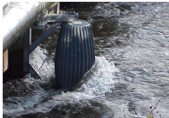
Close up of a debris sweeper installed on the Cedar Creek in Washington.
