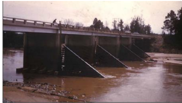
Debris fins independent of bridge pier structure (Bradley et al. 2005)
