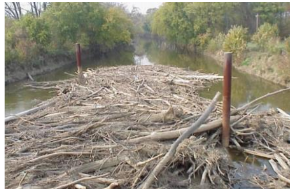
Debris accumulation at single column debris deflectors (Lyn et al. 2003)
