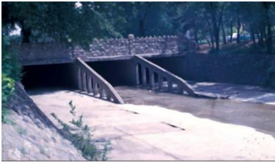
Debris fins upstream of bridge piers (Lagasse et al. 2010)
